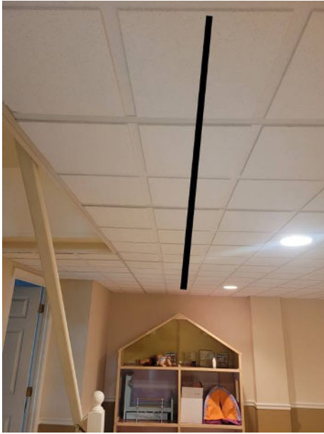
approximate area of floor structure deficiency
